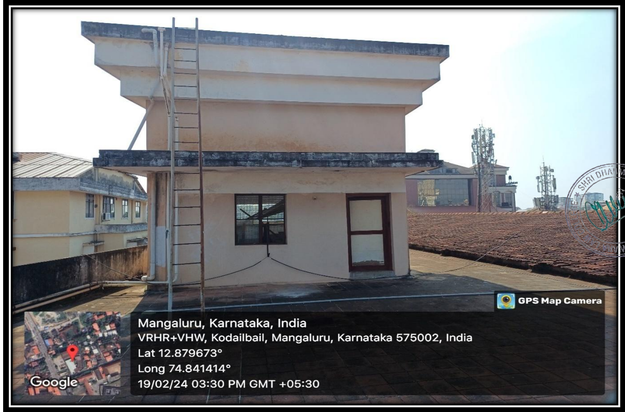
Water Storage Tank with Pipe Connections
